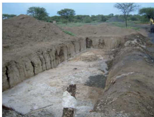
Dumping hole left open for some time – see ground erosion
