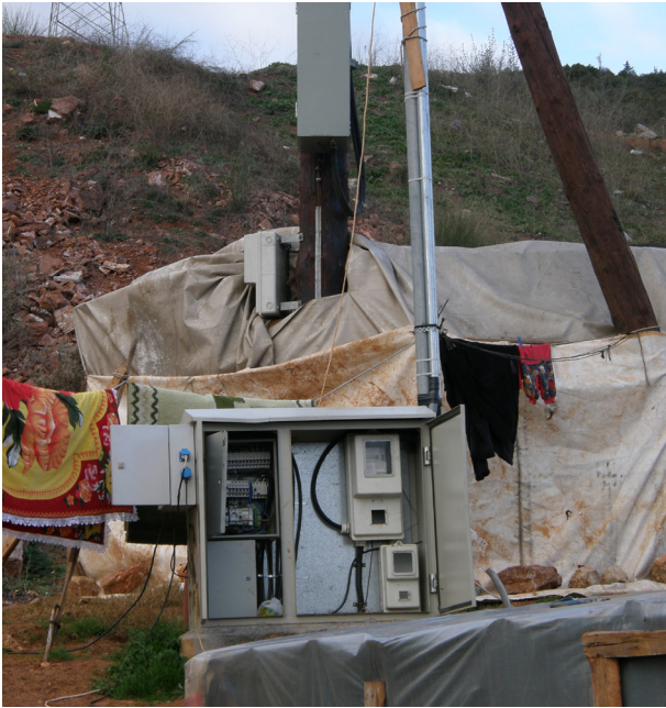
The Roma settlement site in Kamilovrysi in the prefecture of Phthiotis: electricity connections
